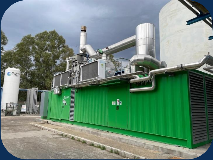
Onsite cogeneration and backup power capacity
